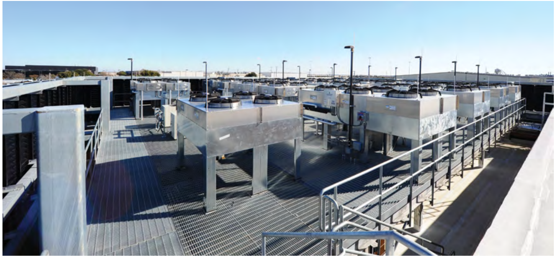
Below ▼ Commissioning helps ensure critical building systems perform as expected
