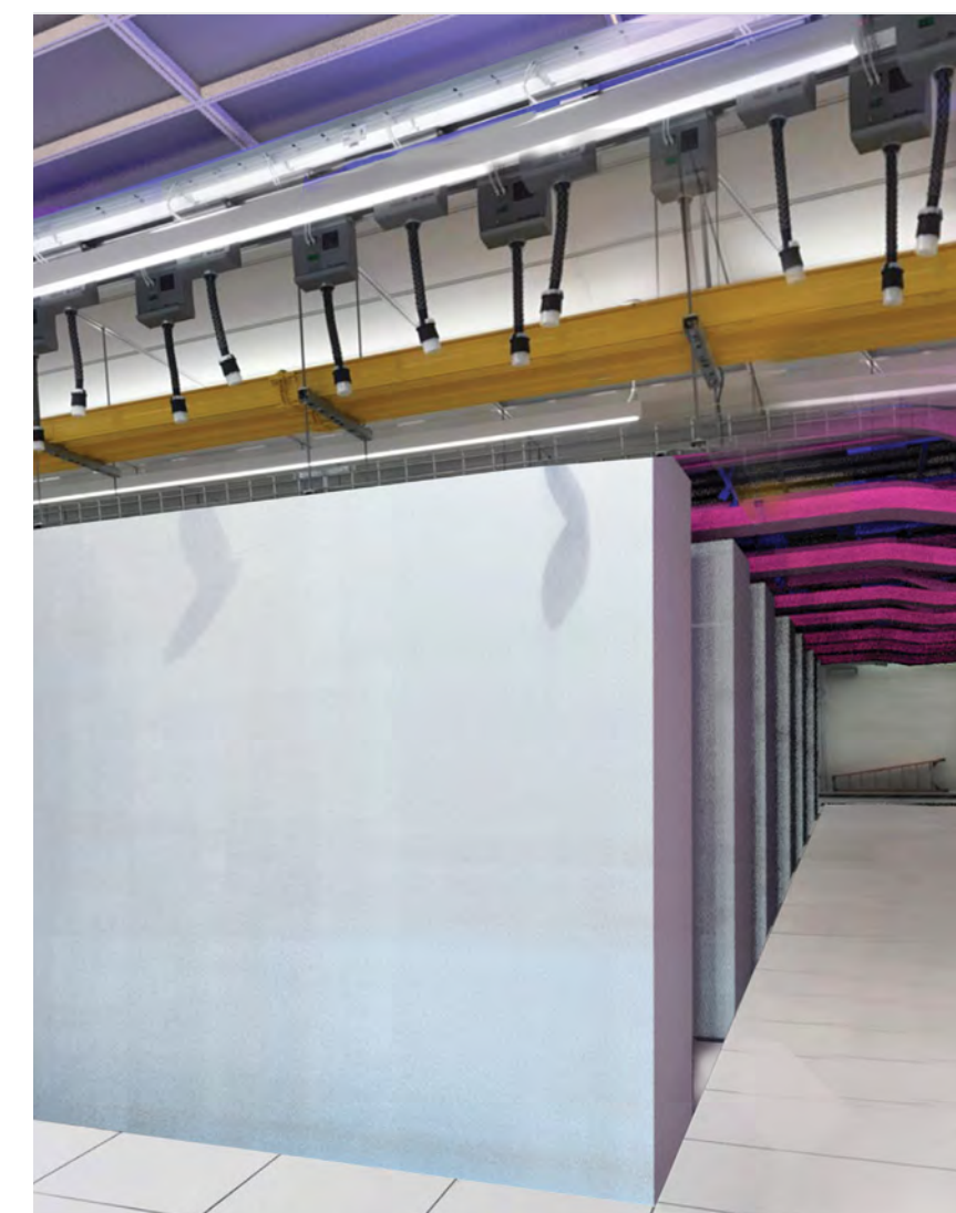
Above ▲ 3D modeling can make sure complex infrastructure fits into the space as designed
