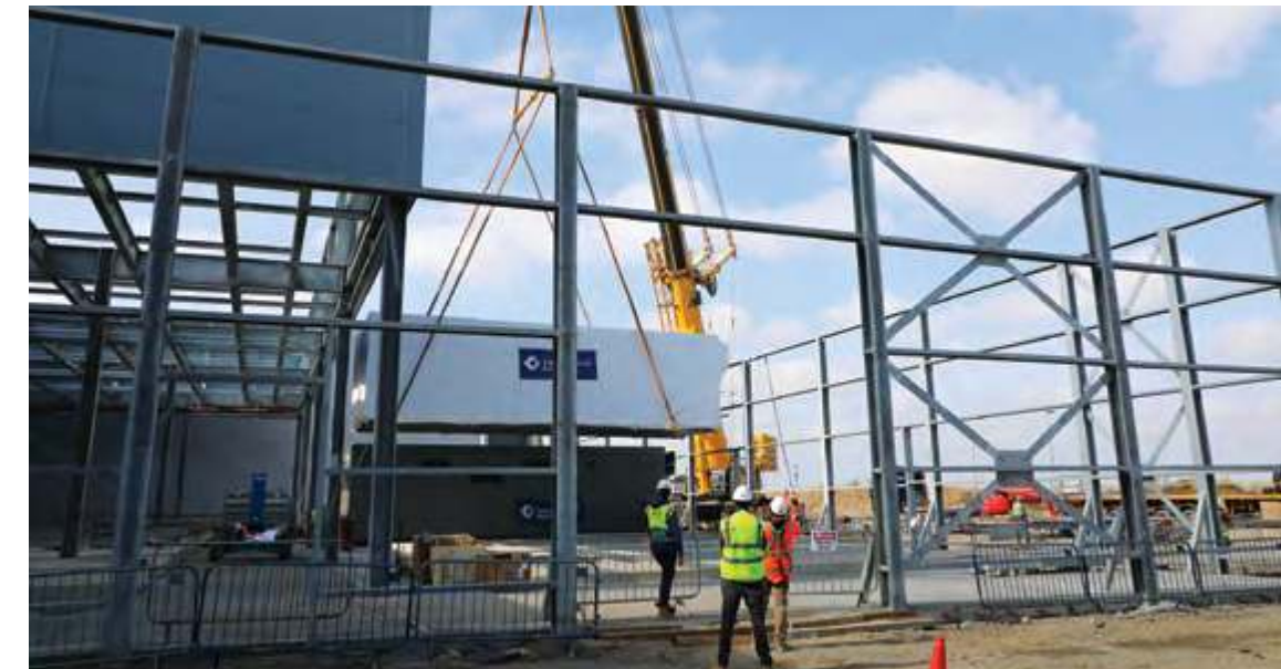
△ The project involves both core-and-shell and interior fit out of the new data centre
