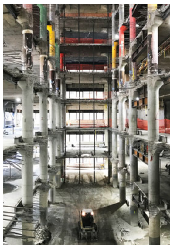
Above ▲ Demolition of existing slabs makes room for a new structural core
