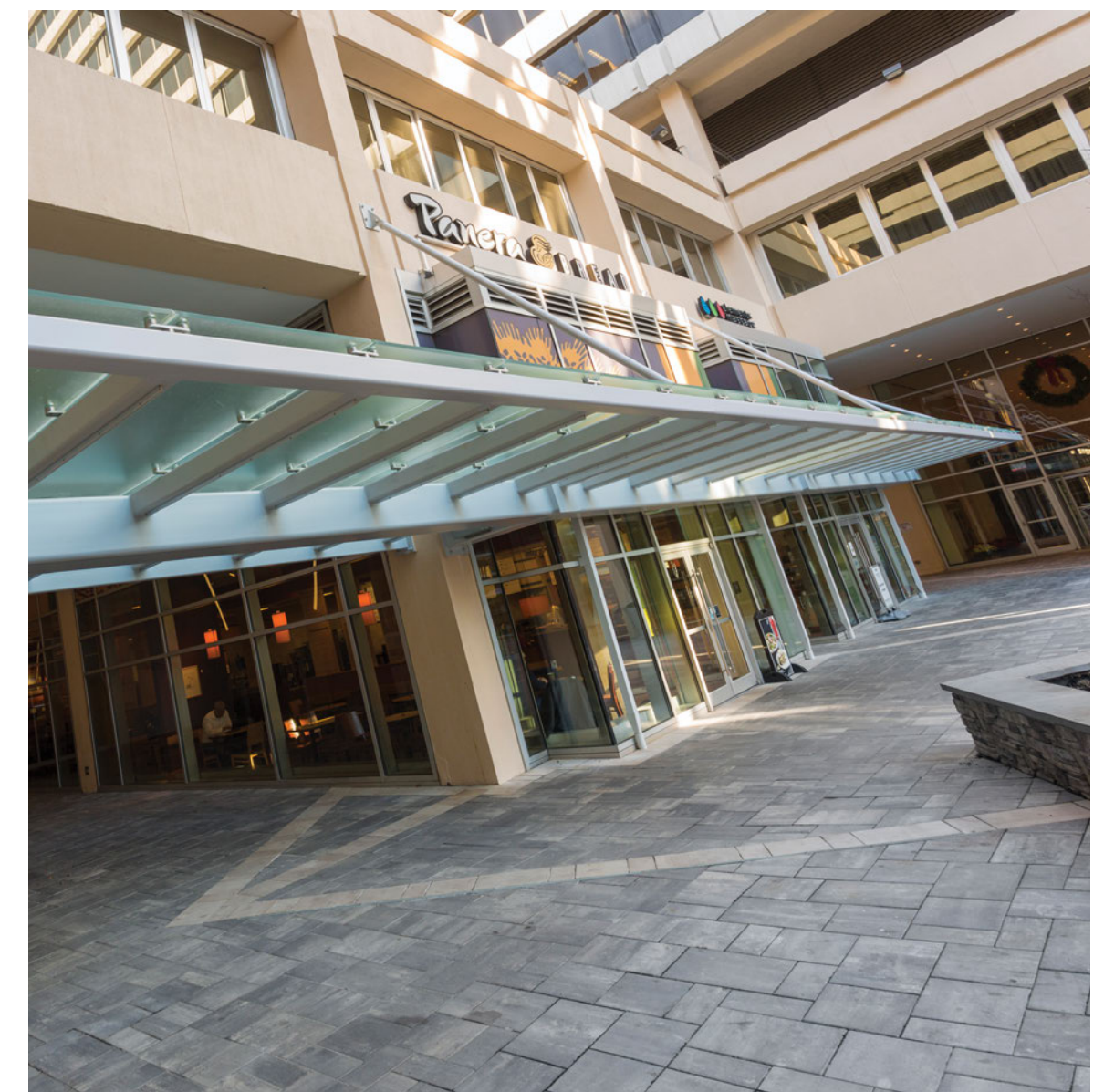
Above ▲ Renovations to the exterior at 1 North Broadway include a new overhang and updated lighting and finishes
